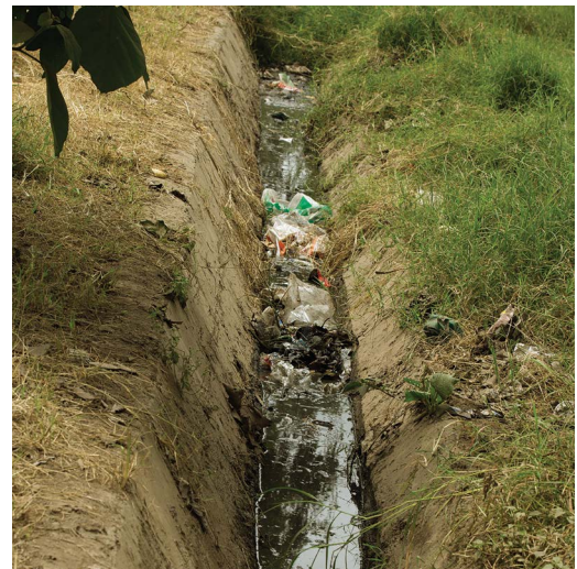
Clogged drain along Muigai Kenyatta Road. © CDKN
